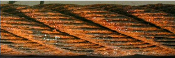
4. Surface badly pitted, wires without tension, gaps between wires. Immediate storage.
