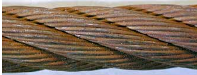
1. Beginning of surface oxidation, can be wiped clean, superficial – Rating: 0% towards discard
